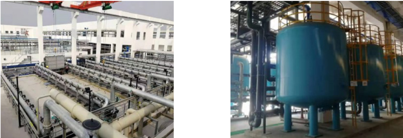
MBR Sewage Treatment Facilities and Activated Carbon Tower Absorption Facilities
